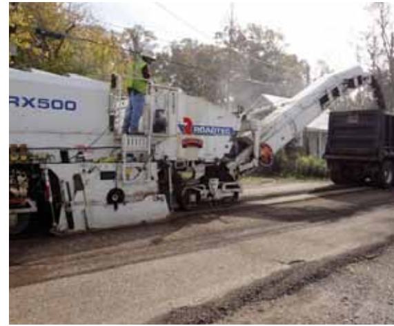
ABOVE LOUIS BABIN, OPERATING BARRIERE'S ROADTEC RX500 MILLING MACHINE IN MANDEVILLE, LA.
